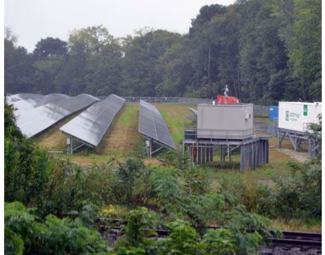
ENGIE North America and Holyoke Gas & Electric: The largest energy storage system (with solar) in Massachusetts, located at the site of the old Mt. Tom power plant.
